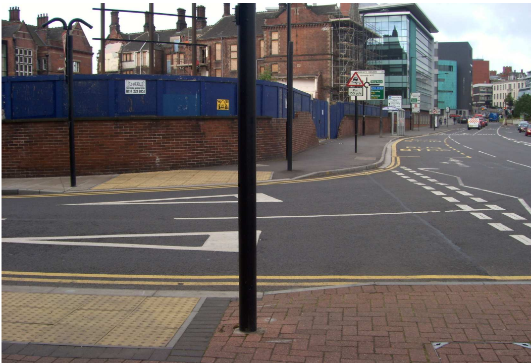
Photograph One: Site of the proposed signal controlled crossing at the junction of St George's Terrace and Broad Lane. The photograph shows that the majority of the civil engineering work associated with the signal controlled crossing was completed (including the poles and ducting for wiring of the signals) before work on site was stopped. A crossing in this location would improve access to the bus stop just visible in the background.
